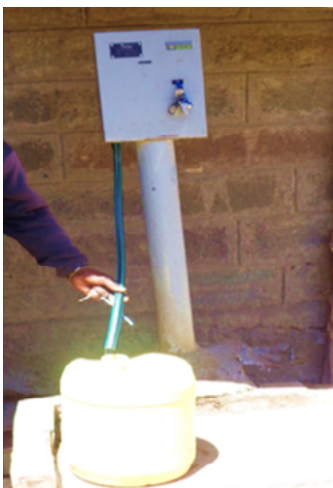
Figure 1. Photo of pre-paid meter
